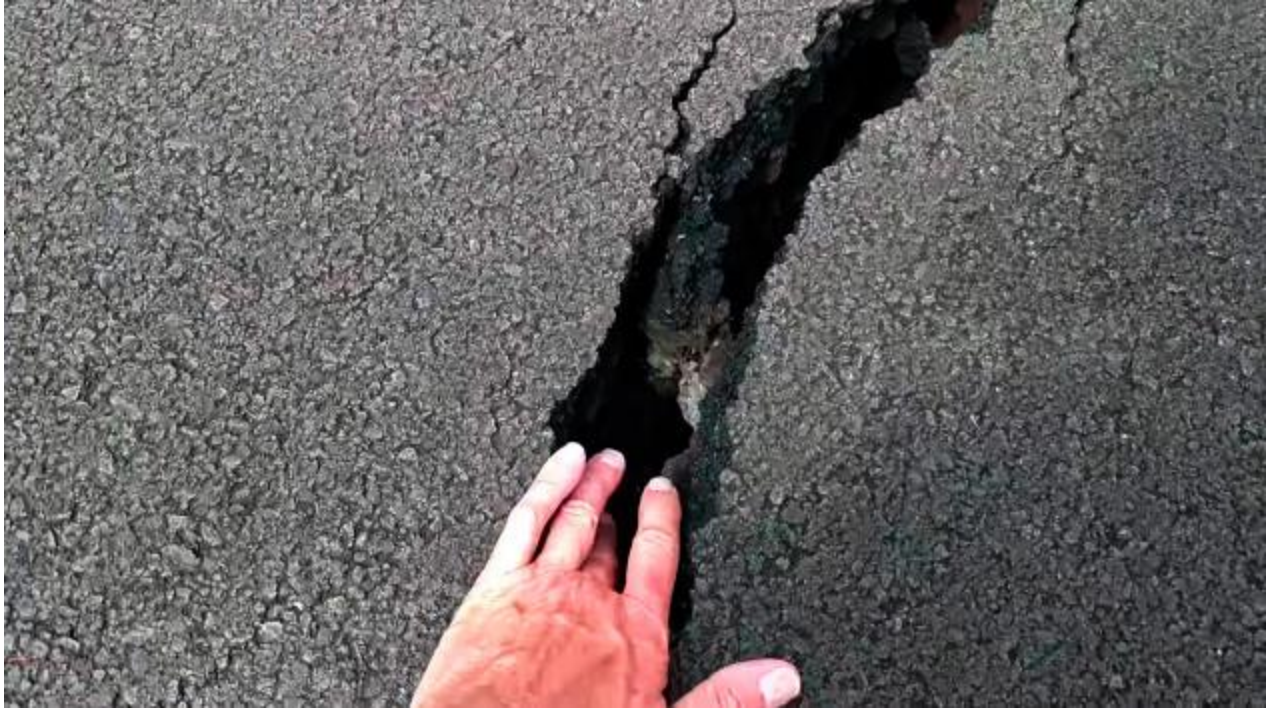
A fissure in a road in the Leilani Estates subdivision. (Scott Wiggers/Apau Hawaii Tours via AP)
